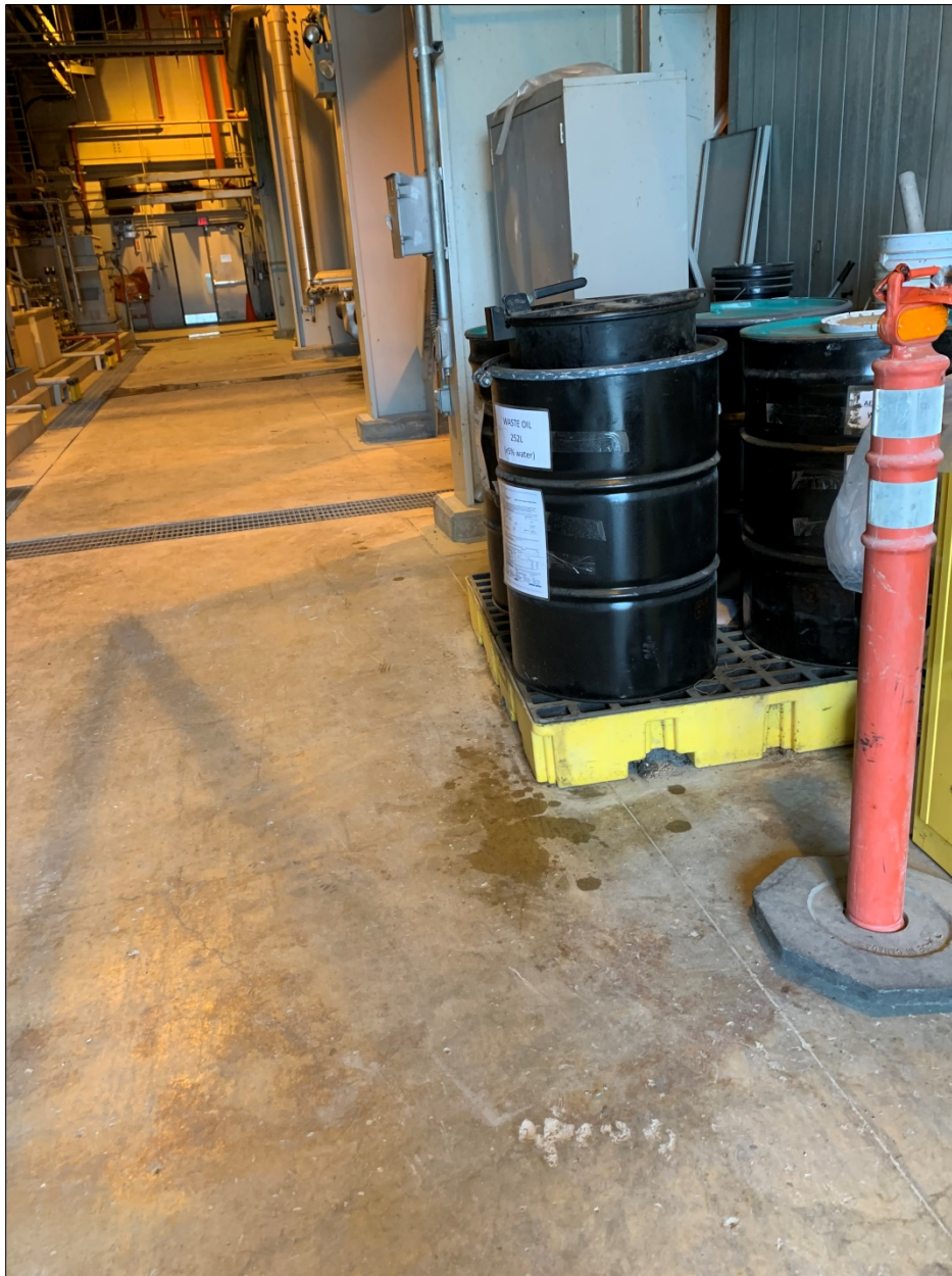
Figure 1: During the virtual site visit, a small quantity of liquid was noted on the floor beside the waste oil drum. The above picture was provided to BluMetric following the audit and was taken after the liquid had been wiped up.
